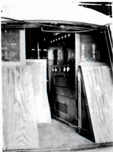
As a part of the equipment appears in the rear of the unit.
